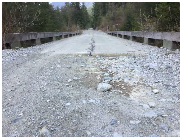
Approaches require surfacing
