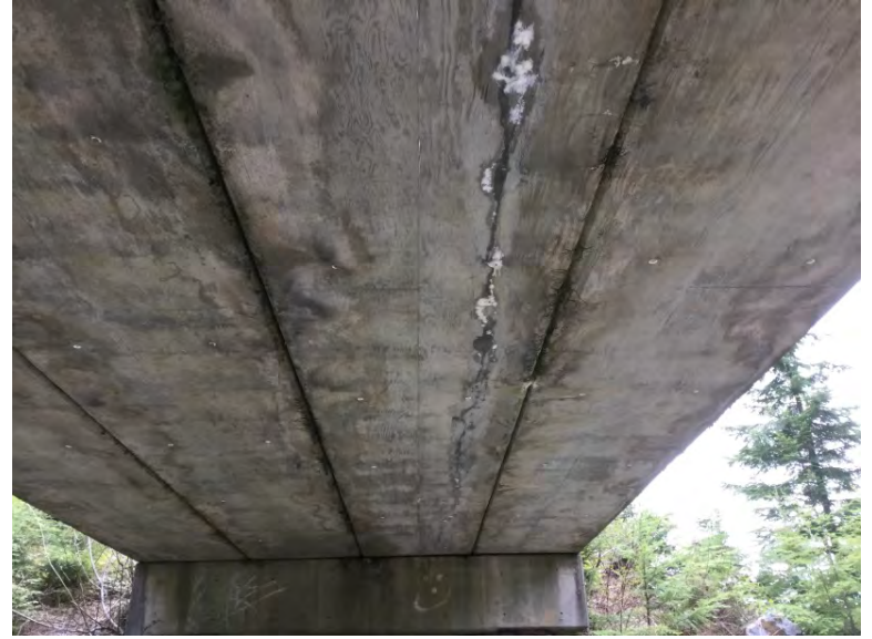
Efflorescence on slab 3
